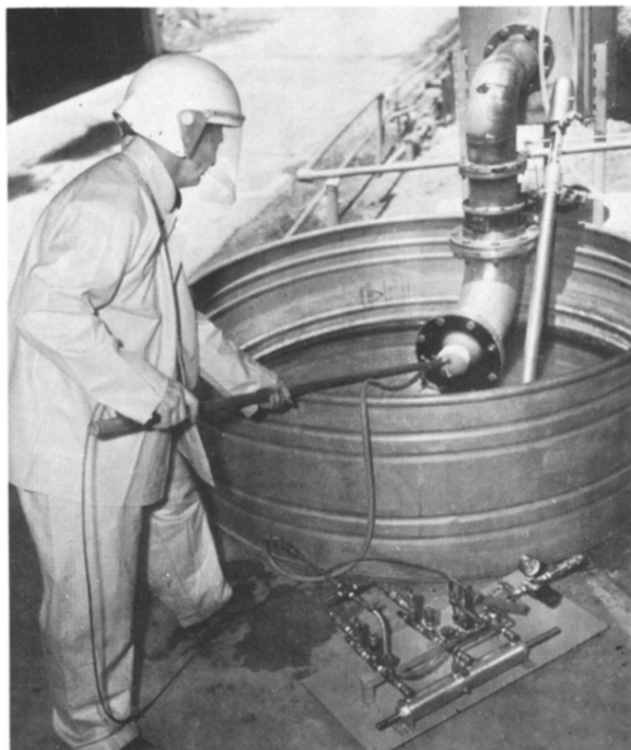
Fig 11 Foamed-in-place leak plugging system showing CO 2 capsule-driven two-component foam generator (lower right), foam-filled plug inserted in “leak” (right-of-center), and operator with control/guide wand (left) System is being assembled as a back-pack unit The equipment (upper right, above tank) controls head and flow rate of “leak” during testing
