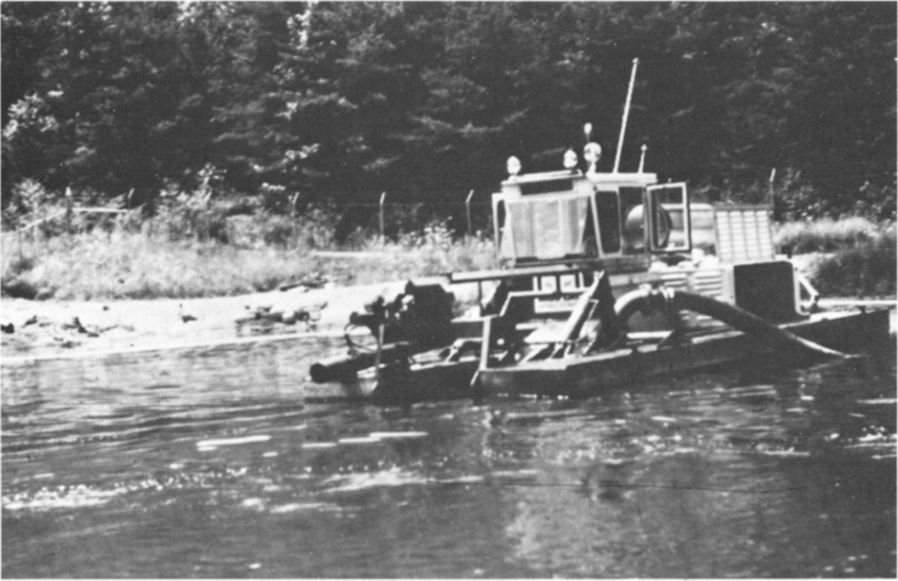
Fig 7 Pontoon-mounted vacuum dredge in use to remove contaminated silt from pond bottom showing (from left to right) towing winch, control arms for submerged auger, cabin, effluent hose, and diesel engine Effluent line is supported by air-filled bags and is arranged in a snake-like configuration on pond Nominal pumping rate is 1500 gal/min of 20% slurry.
